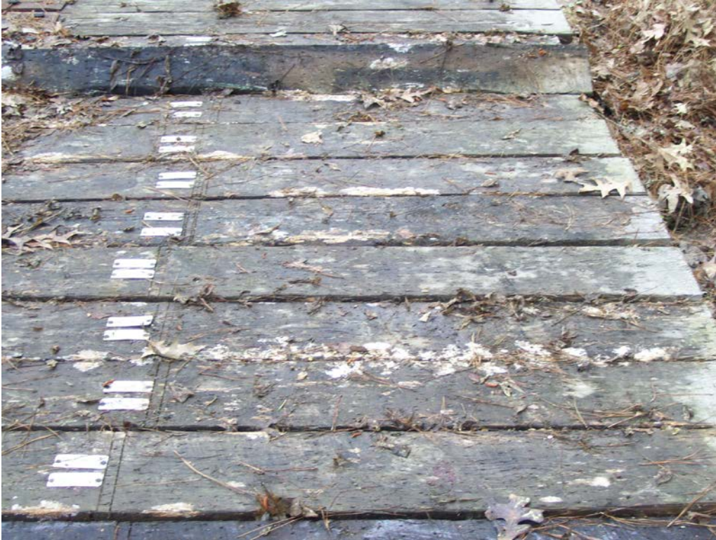
Figure 4 - Untreated white oak ties with mycelium or signs of decay.
