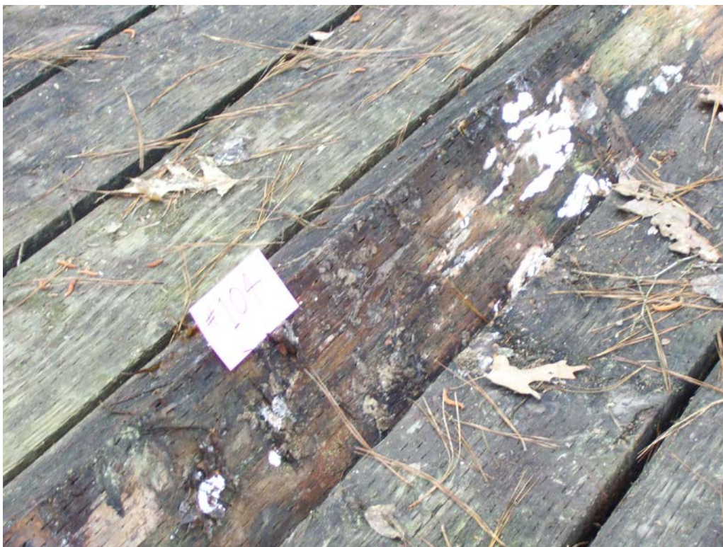
Figure 3 - Tie #104 showing trace amounts of decay.
