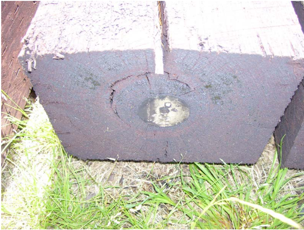
Figure 6 - Tie #191 with check and ring shake.
