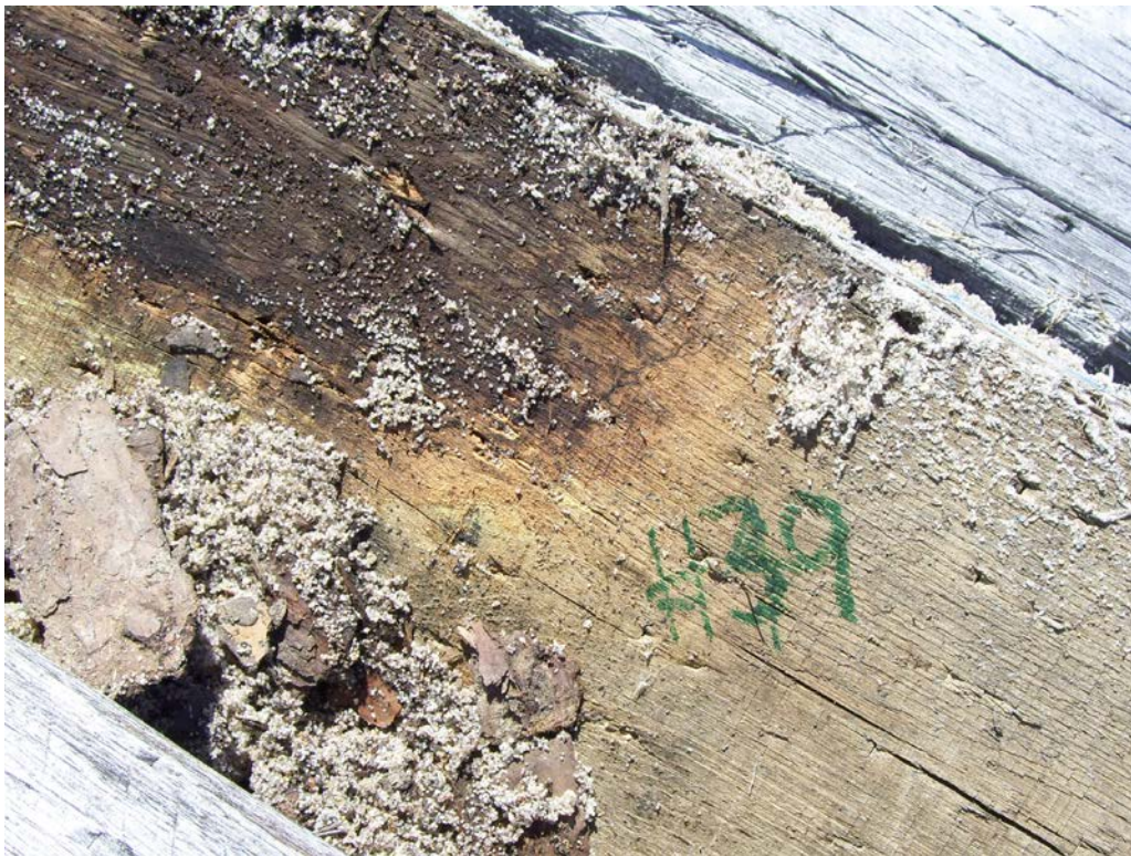
Figure 7 - Tie #39 with slight decay and trace termite damage.
