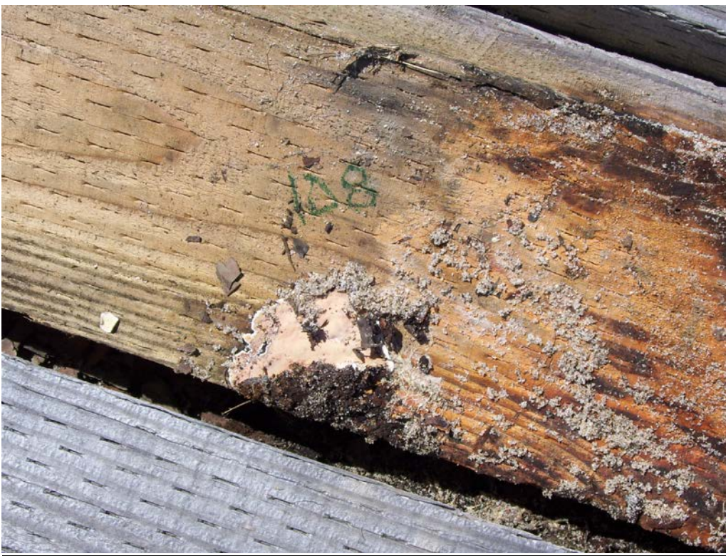
Figure 5 - Tie #108 (D-fir untreated) with light decay.
